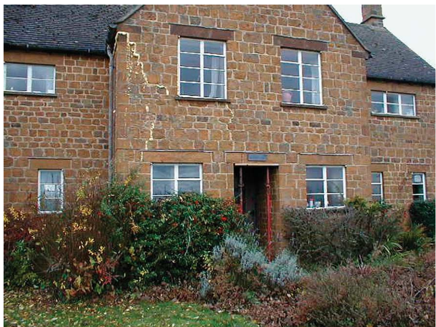
Figure 2: Severe cracking to a sandstone house in Oxfordshire caused by fruit trees growing in the garden (note the foam filling in the cracks and the jacks supporting the lintel)
